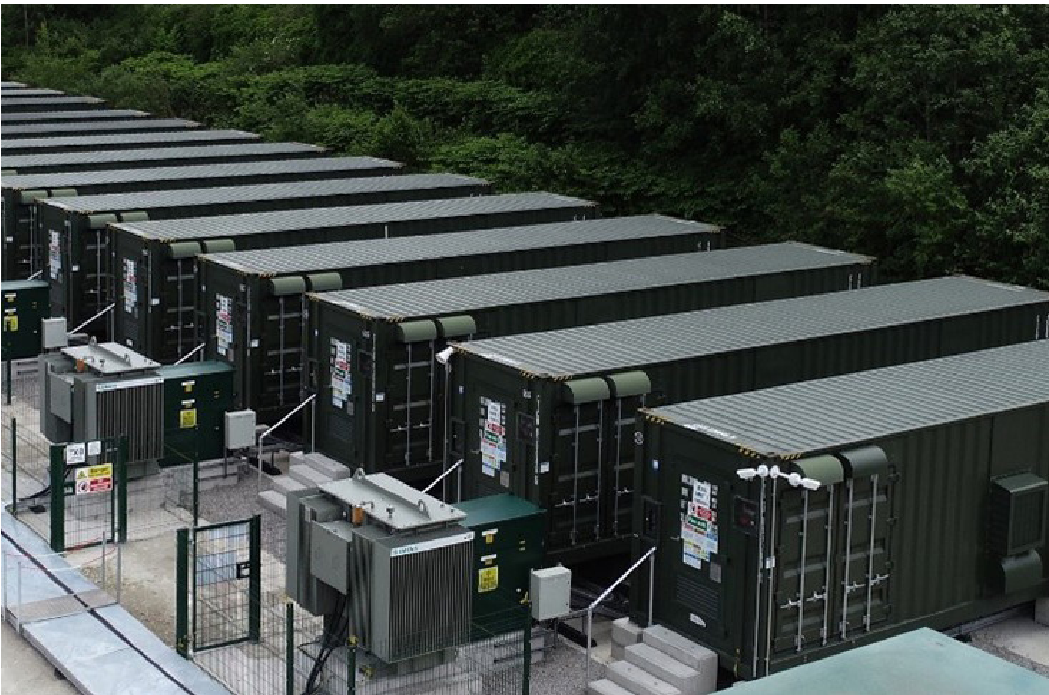
Example Battery Storage facility
